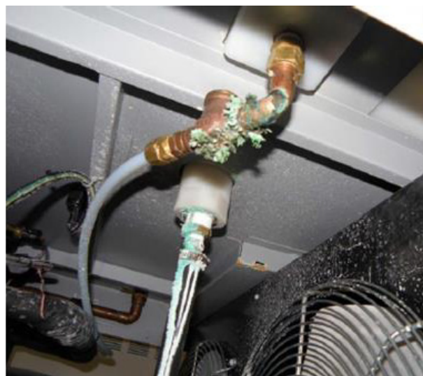
Figure 4: Corroded chiller fittings on AES Baseline tool.
